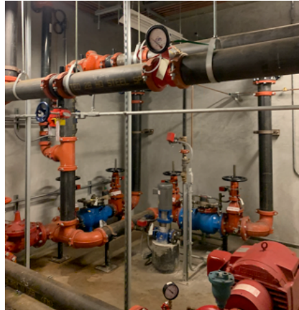
Fire pump room at basement
