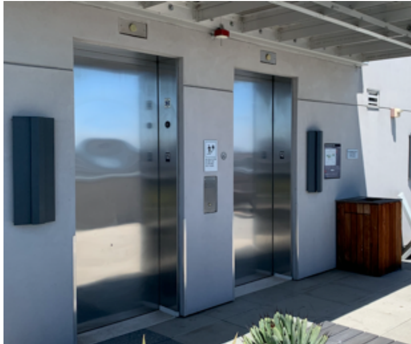
Lighting at elevators at the roof deck
