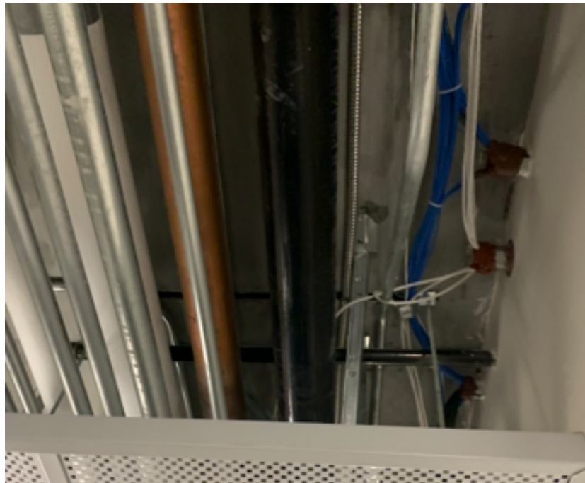
Building piping as seen at hallway ceiling - copper water supply, cast iron waste
