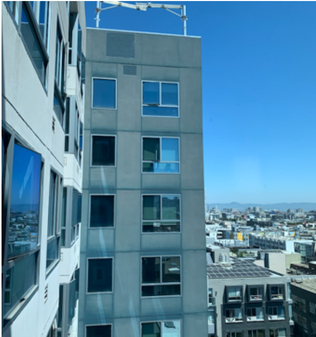
West facing side of south building section – EIFS panels faded
