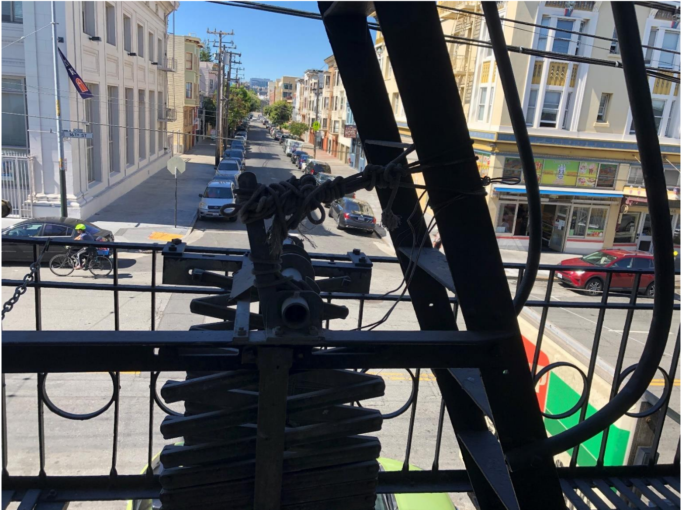
Photo 6. Nonfunctioning fire escape
