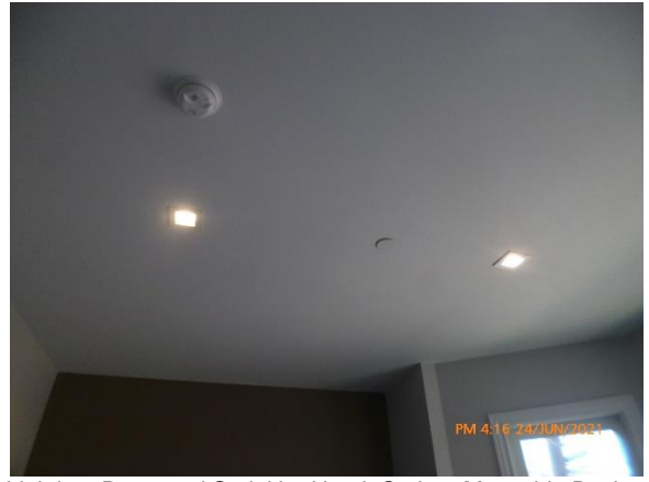
Lighting, Recessed Sprinkler Head, Carbon Monoxide Device
