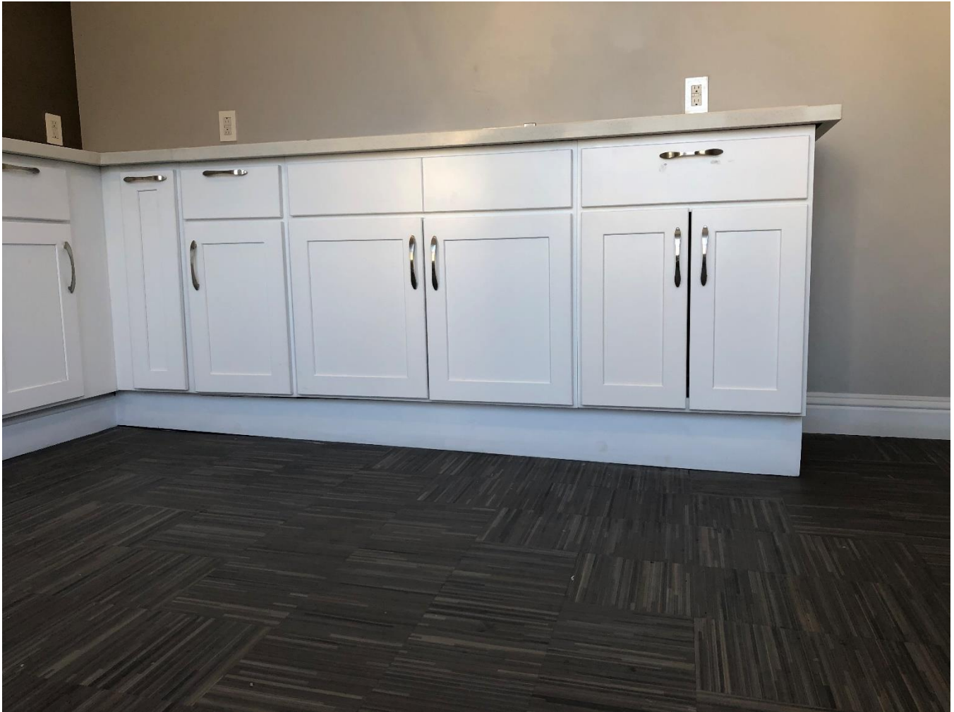
Photo 4. Sloped floor at kitchen counter
