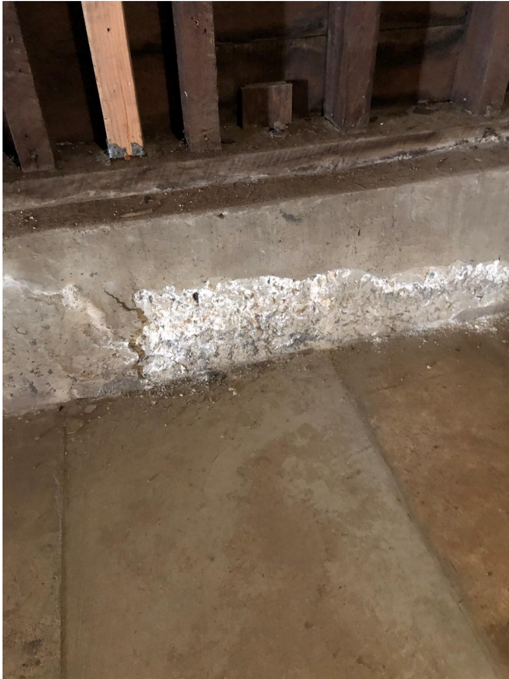
Photo 5. Deteriorated concrete in the basement footing
