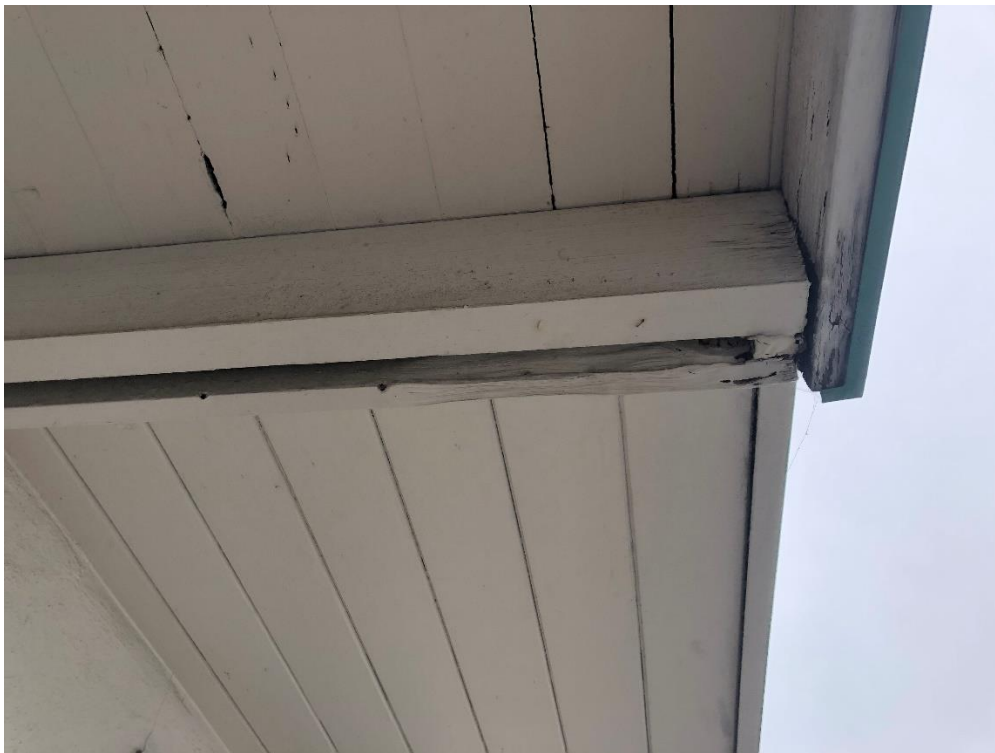
Photo 4. Damaged beam at Building B exterior walkway
