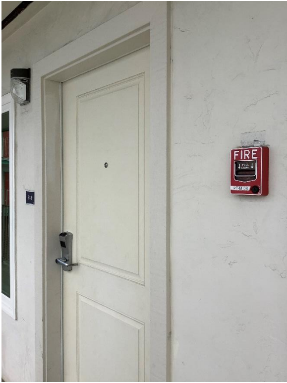
Motel room Entry Door with Card Reader
