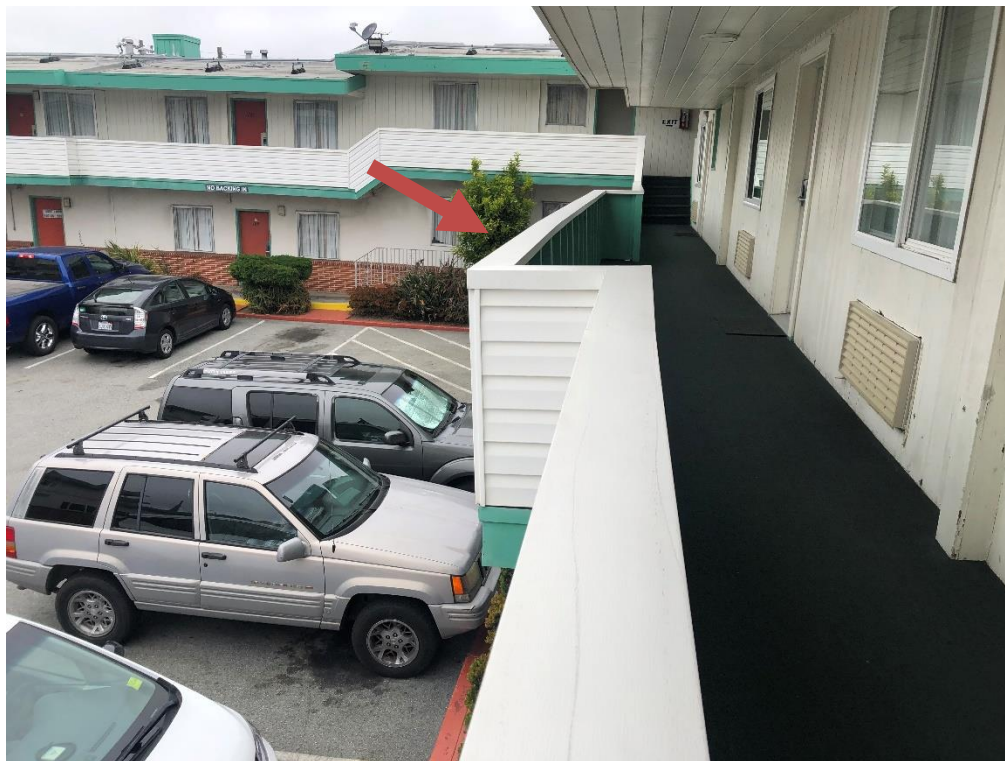
Photo 6. Damaged/loose guard rail at Building B
