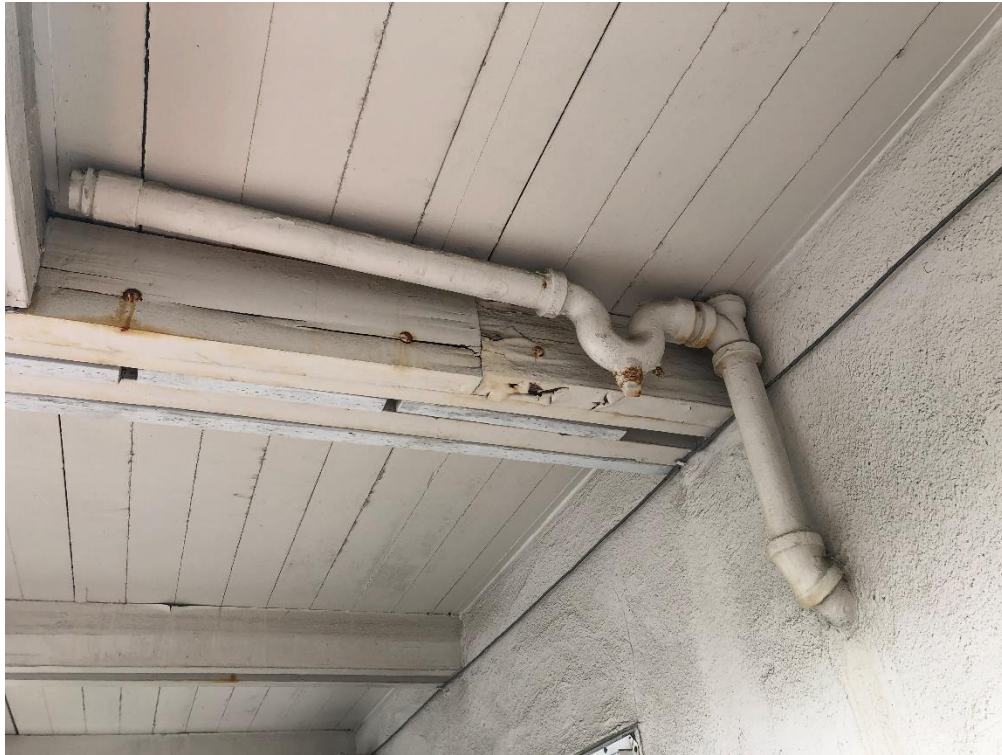
Photo 5. Previous repair at damaged beam at Building B exterior walkway
