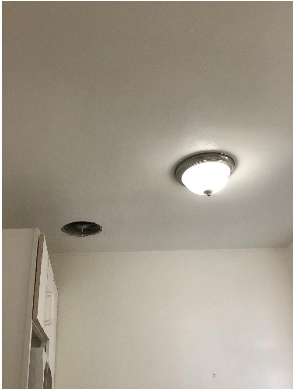
Exhaust, Lighting, Upper cabinet in non-renovated motel room
