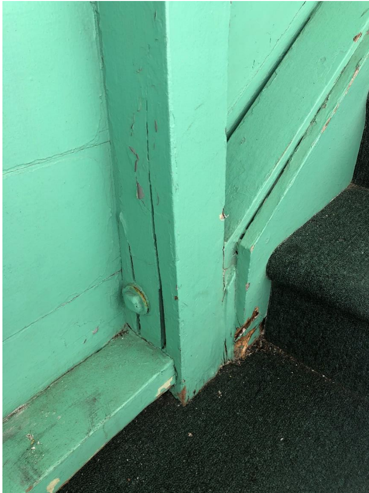
Photo 7. Damaged post at Building B guard rail
