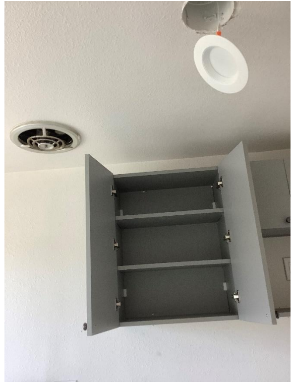
Exhaust Fan, Recessed Light, Upper Cabinet in renovated motel room.
