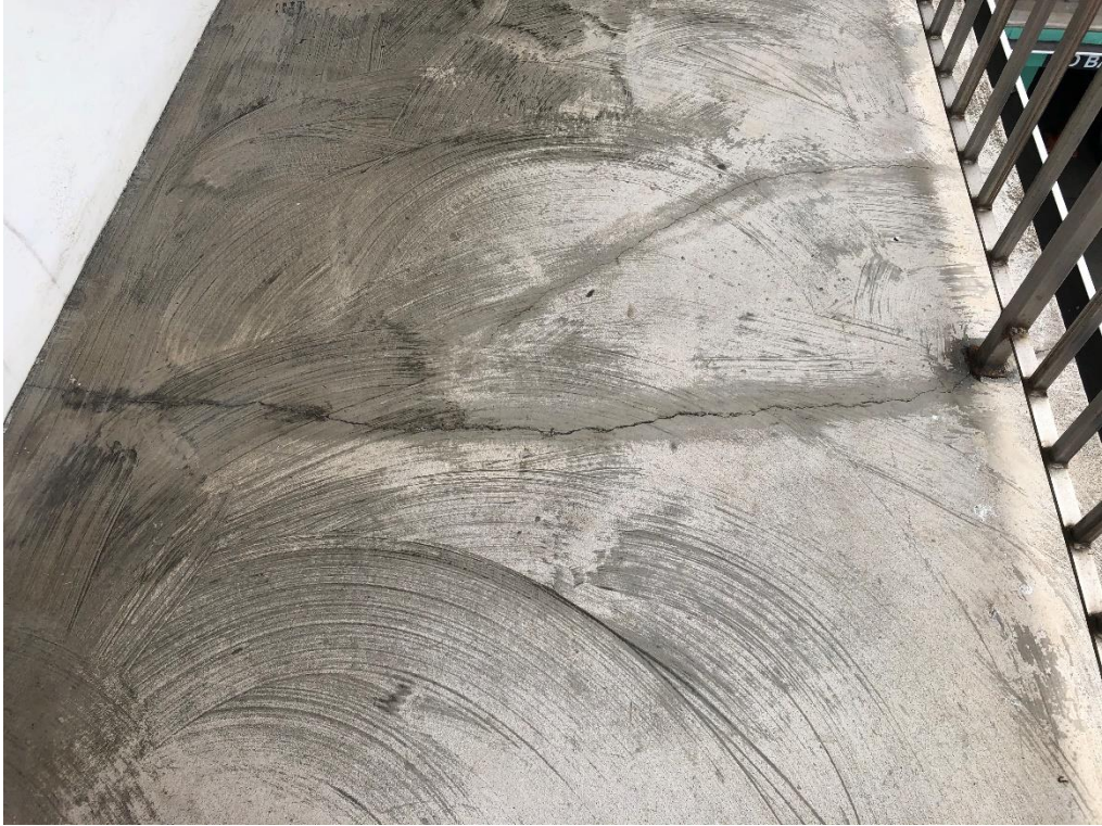
Photo 8. Cracked topping slab at Building A
