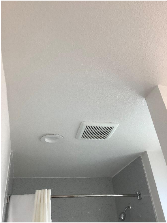
Bathroom Exhaust Fan, Lighting in renovated motel room
