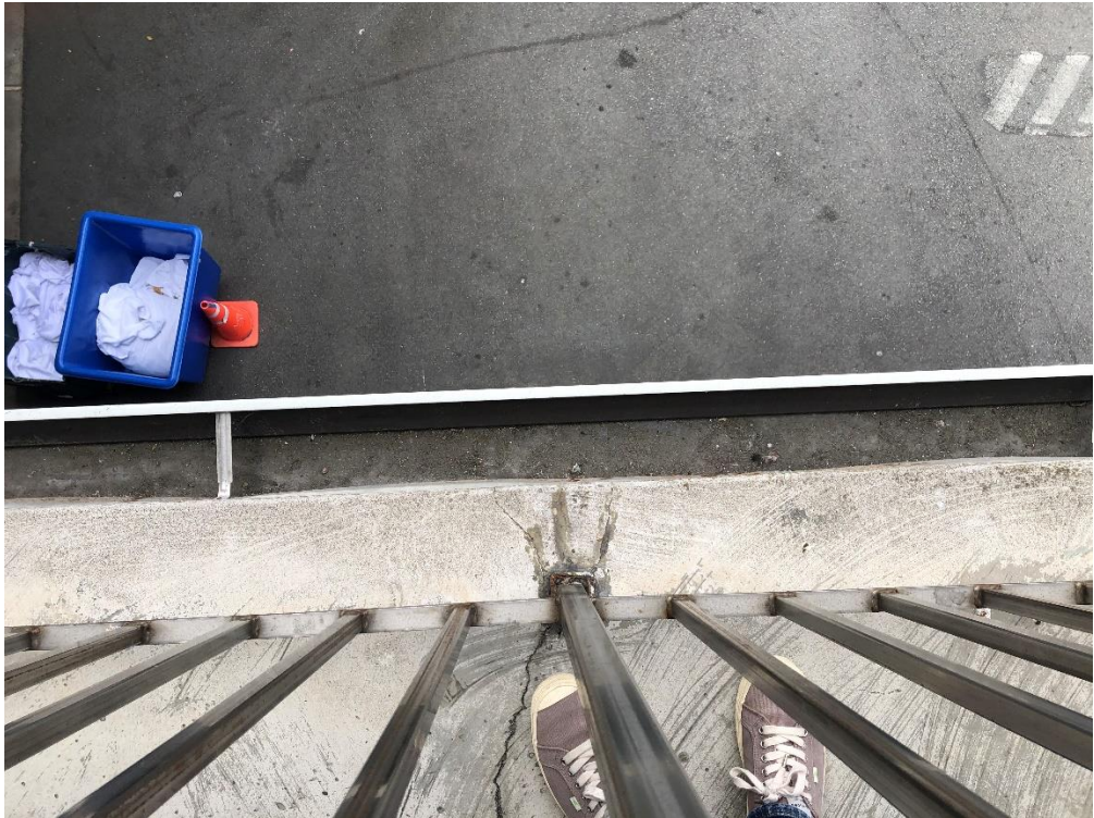
Photo 9. Cracked topping slab at Building A
