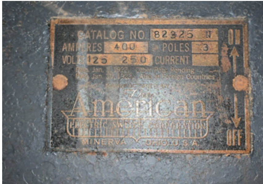
Original tag on breaker cover
