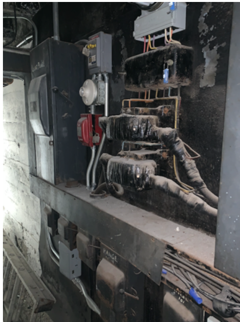
Main and various subpanels. Newer meter above.
