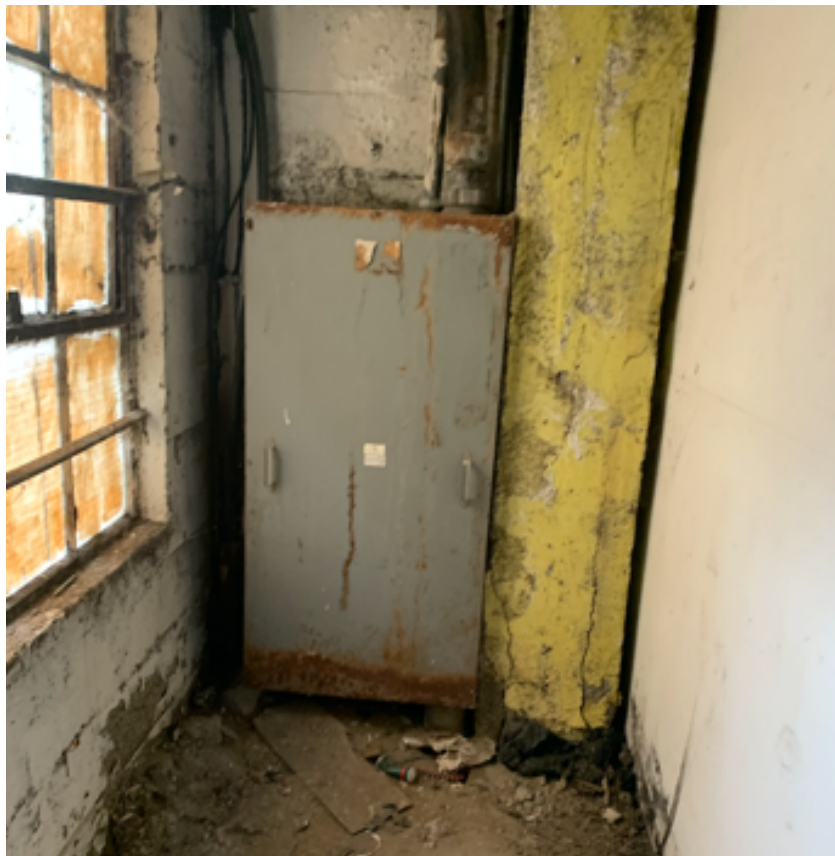
Stressed concrete post at upper garage (east side) near electrical switchgear
