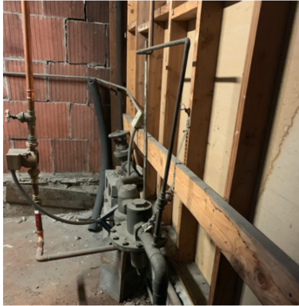
Terra cotta wall and crumbling footing wall – observed at boiler room – upper garage
