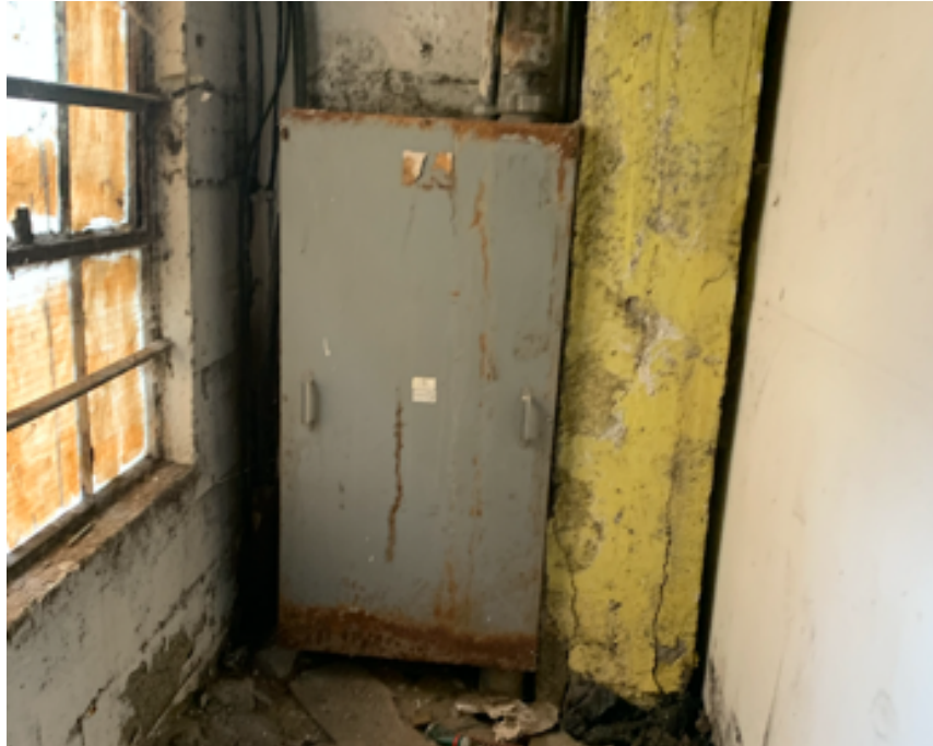
Transformer / service entry container at electrical switchgear area. No information as to whether this is online or not was ascertained. The tag was worn off.
