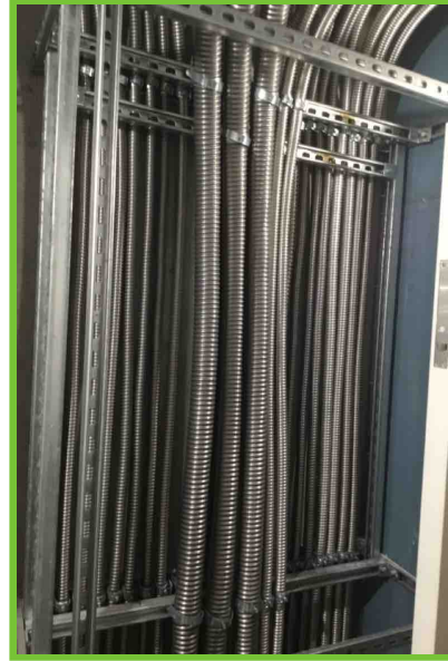
Note: 7th floor electrical
