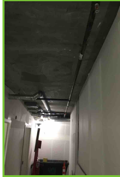
Note: Office mechanicals
