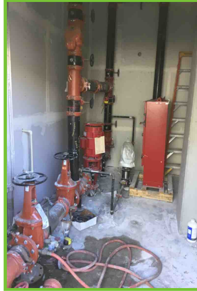
Note: Fire pump room
