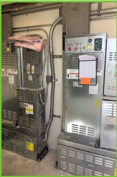
Note: Elevator control room
