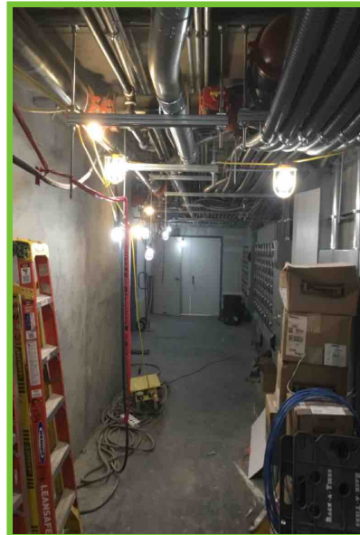
Note: Basement entrance into switch room
