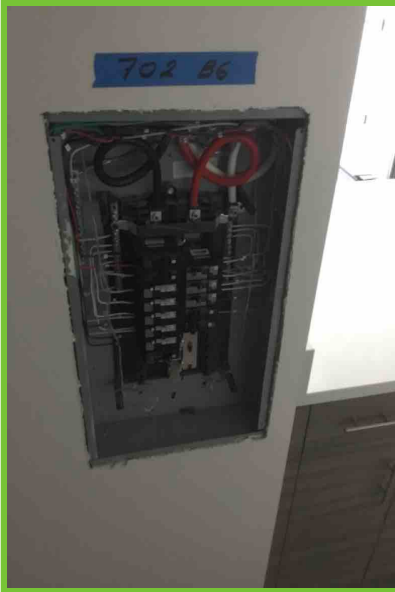
Note: 792 electrical panel
