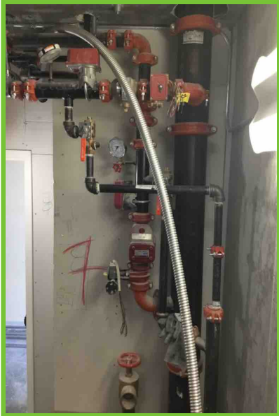
Note: 7th floor Fire controls
