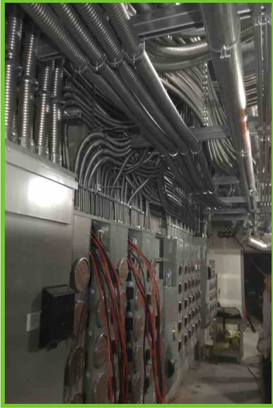
Note: Electrical meter room 2
