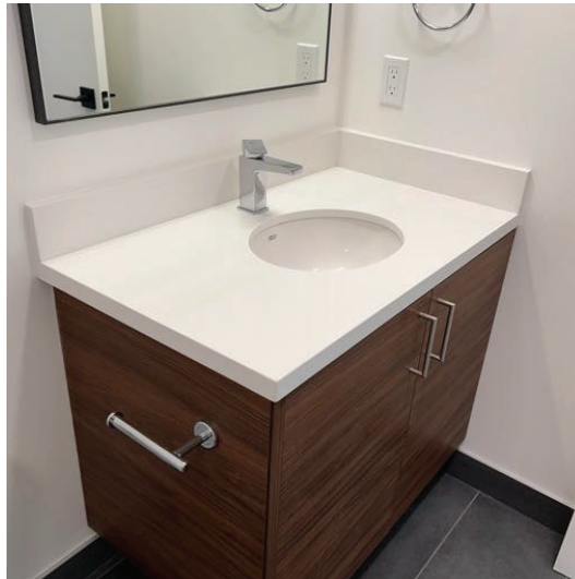
Vanity cabinet, sink and faucet
