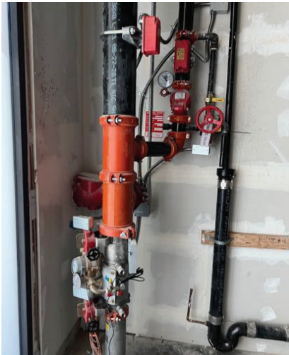
Main backflow at ground floor commercial space
