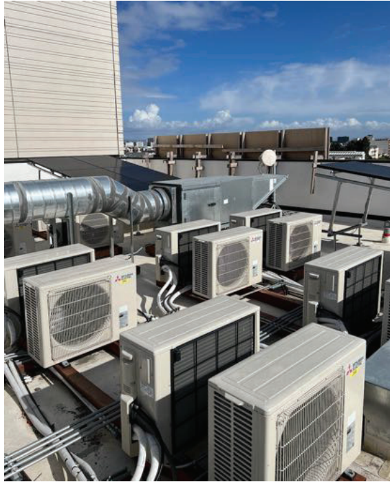
Heat pumps at roof
