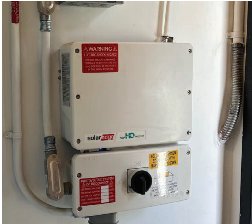
Solar inverter and disconnect
