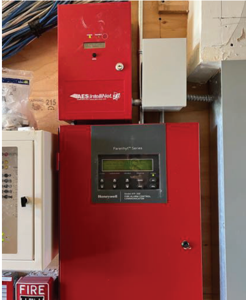
Fire alarm panel
