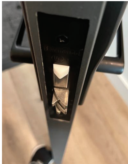
Entry door lock
