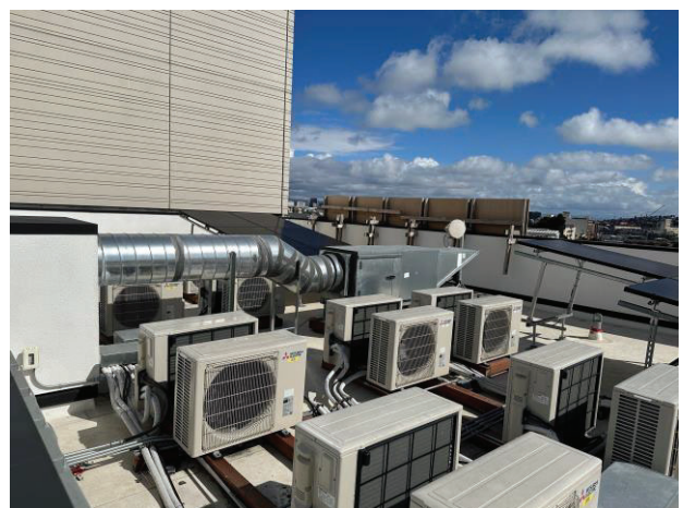
Mechanical Equipment on Roof
