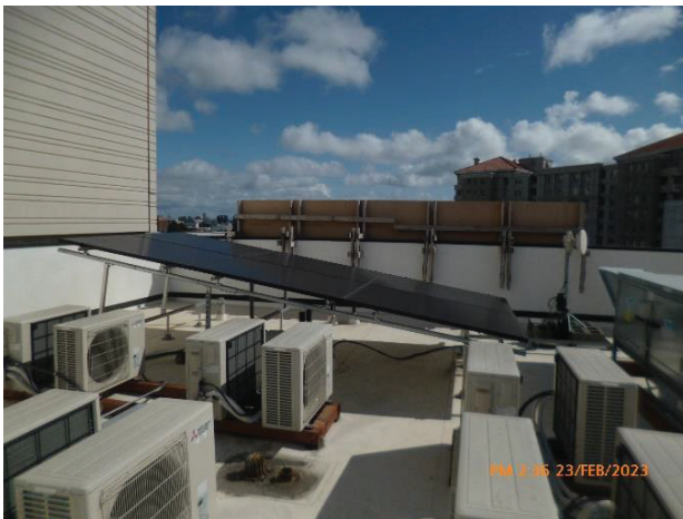
Solar PV Panel on Roof
