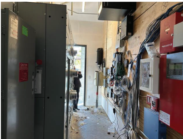
Interior of Electrical and FACP room
