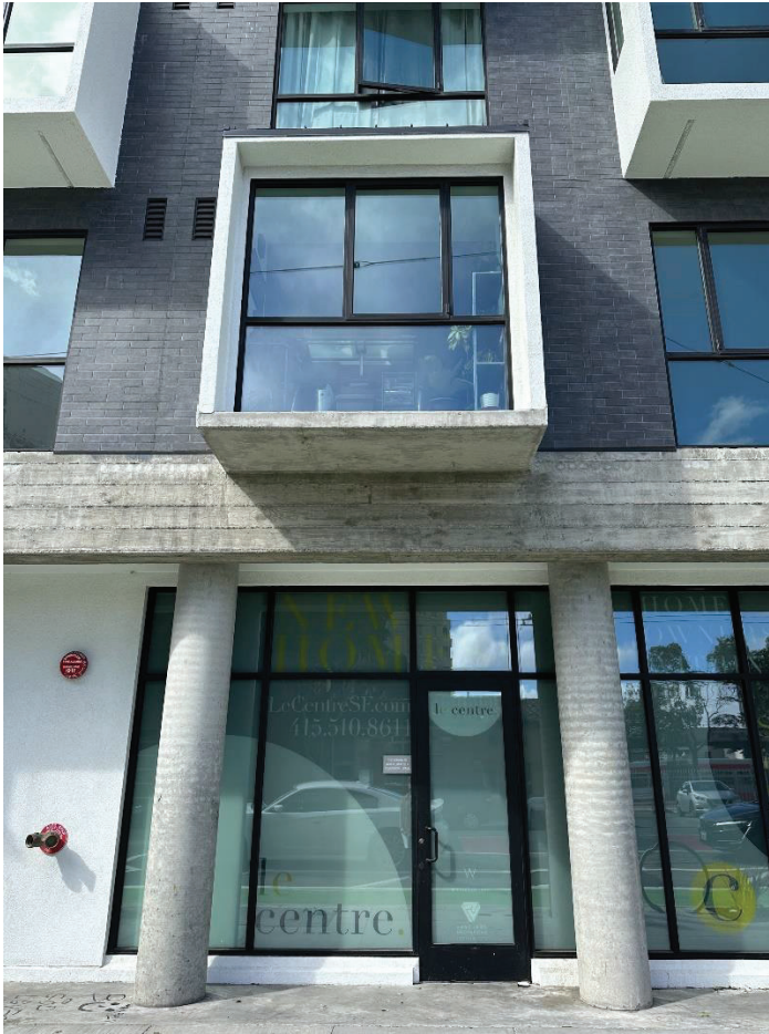
Unit Aluminum Window Assembly and ground floor Storefront System for Commercial Space
