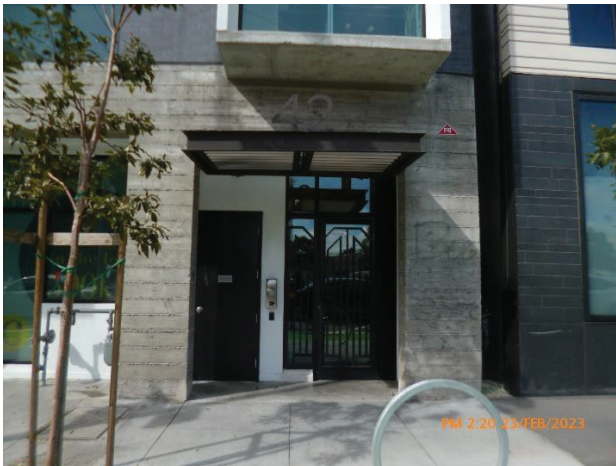
Electrical/FACP Door and Residential Building Entry Door
